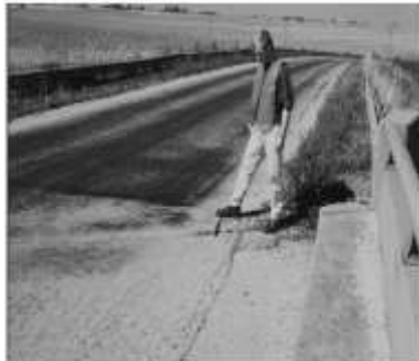
Figure.7.14 Low-Severity Shoving Severity Shoving
