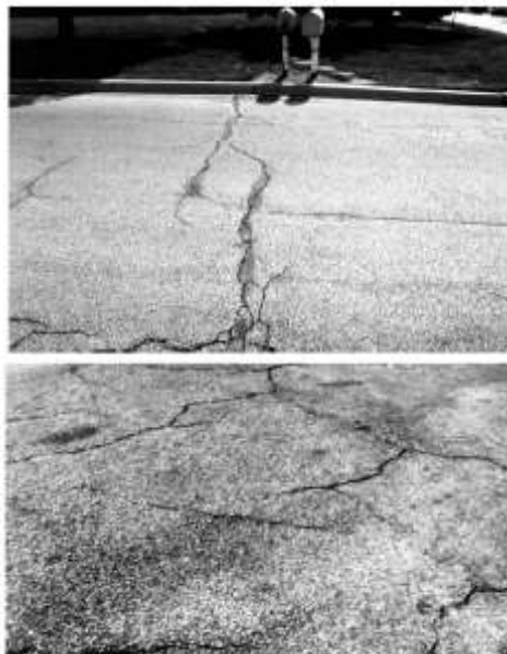
Figure.7.8 Medium-Severity Block Cracking - Figure.7.9 High-Severity Block Cracking
