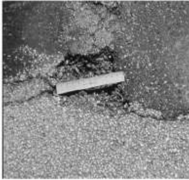
Figure.7.12 Low-Severity Pothole Severity Pothole Source: ASTM (2007)
