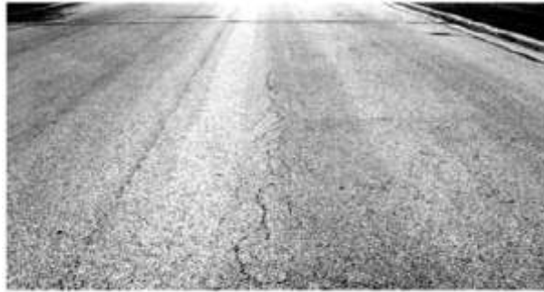
Figure.7.1 Low-Severity Block Cracking Source: ASTM (2007)
